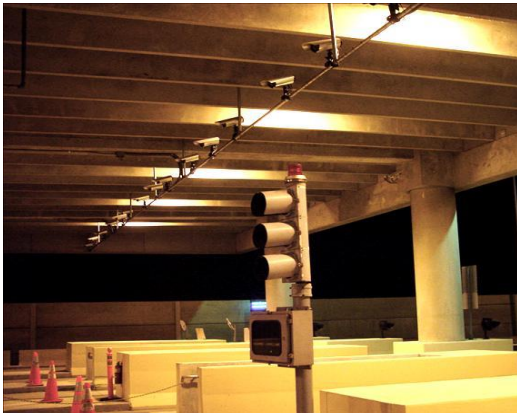
IZTOLL VES Solution Deployed In An ORT System In Florida
