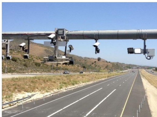
IZTOLL VES Solution Deployed In An ORT System In California
