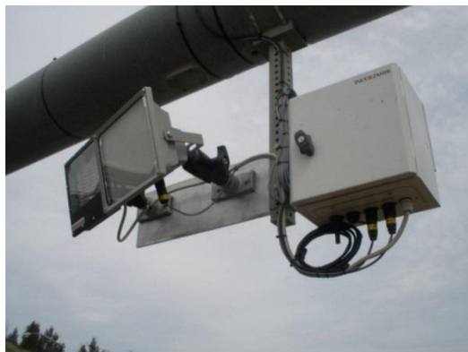
IZODPU Installed At An Open Road Tolling Gantry In California
